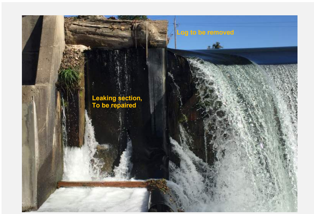
Figure A1-3: Leak creating false attraction flow at fish ladder (10/10/2019)
