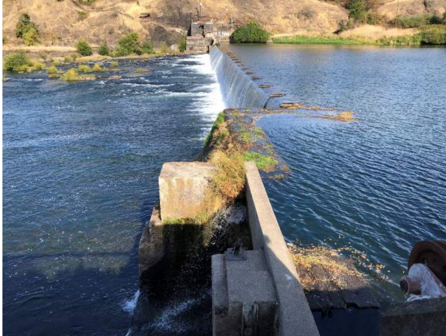
Photograph 1: View looking north across the Winchester Dam from the south power station. (September 2021)
