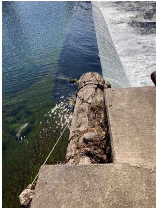
Photograph 4: Log flow diverter on the north side of the dam near the fish ladder. (September 2021)
