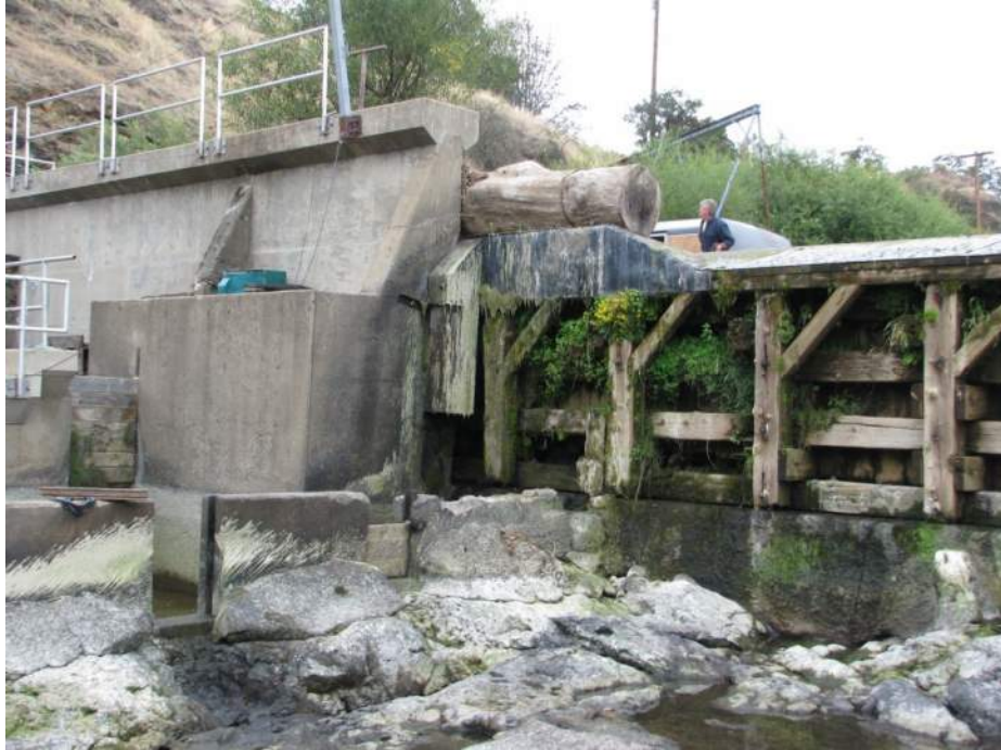
Photograph 6: View of the dam face near the fish ladder where the false attractant flows occur, taken when water levels were previously lowered. (September 2009)
